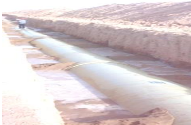
Figure (6) - Flooding of the earthen layer around the pipe
