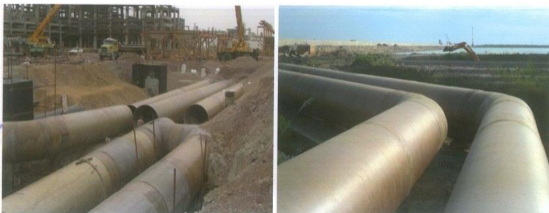
Image (1) A view of the implementation of GRP pipes in industrial projects
