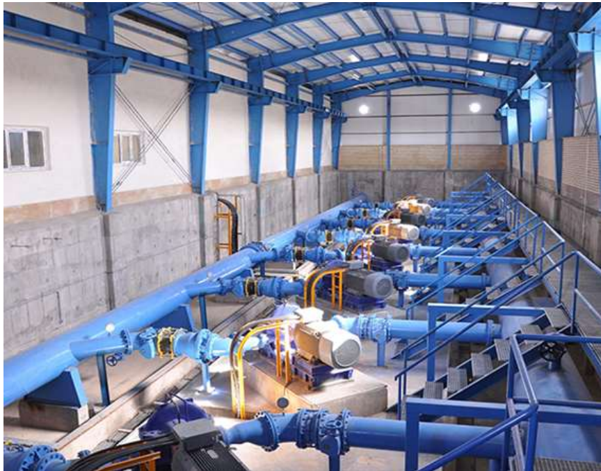
Figure 1. Pumping stations with horizontal pumps.
